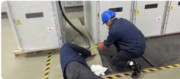
Jinzhai Gotion Electric Shock Accident Emergency Disposal Drill
